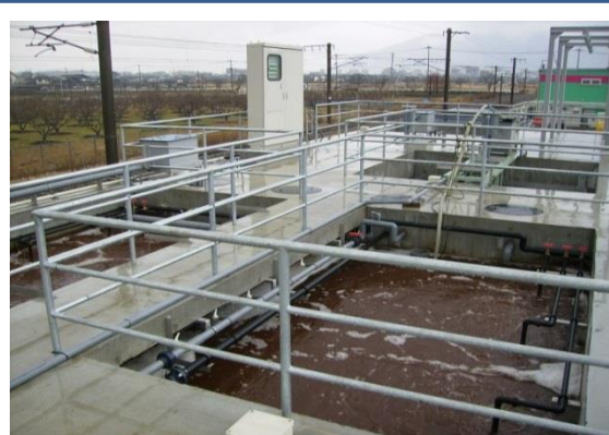
New construction. FR:60ton/day In 2012 (Food processing company)
